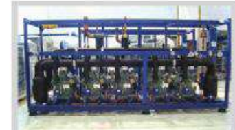
Compressor rack system
